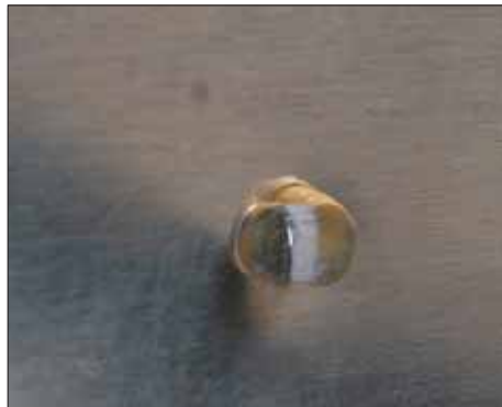
Ouch! The set must have slid off the rivet head on the other side, because the set on this side only hit part of the rivet. Pretty ugly, and this needs to be drilled out for sure!
