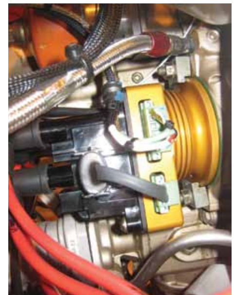
Wiring to an electronic ignition can vibrate over time, leading to failure. Adding Adel clamps will increase reliability.
